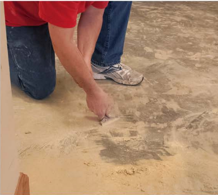
Removing mastic and glue when updating flooring can be a time-intensive process if manual scraping is required.
